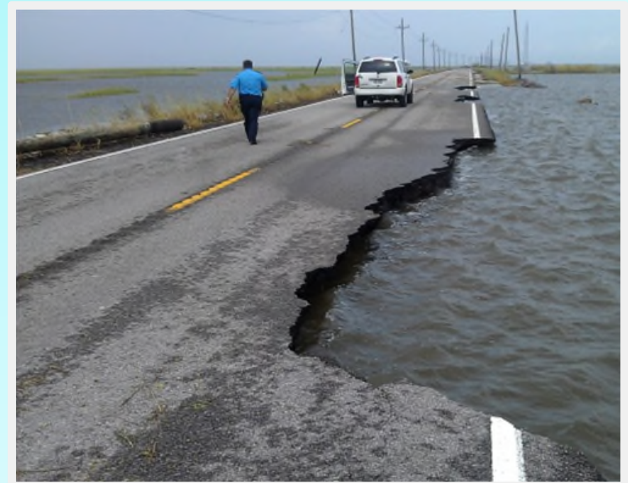
After Hurricane Isaac (2012) Courtesy of LA-1 Coalition
