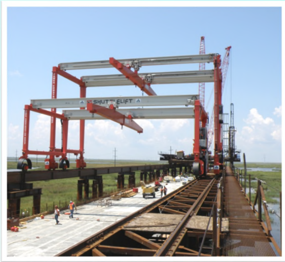
Gantry Cranes and Rail System
